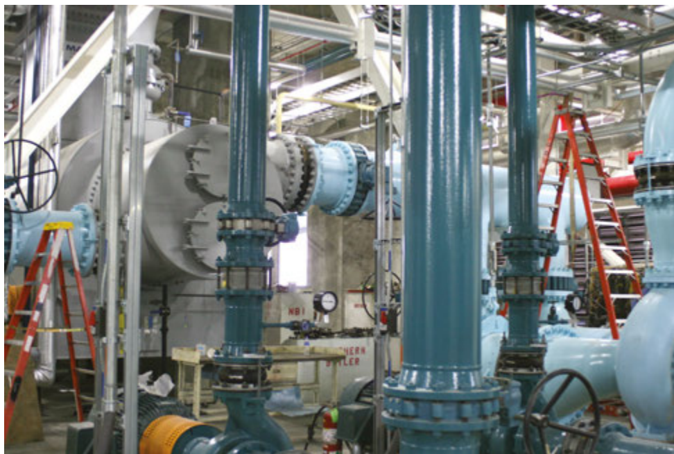
Inside the labyrinth of pipes and boilers at BWL's new $182 million, natural gas-powered cogeneration power plant in REO Town.
